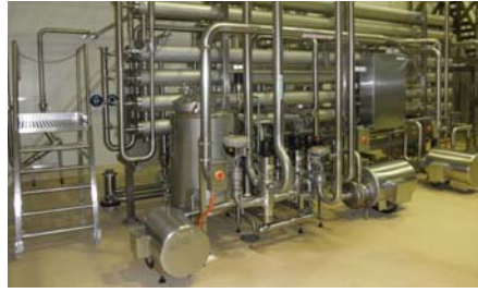
RO plant for water recovery (Courtesy Environment Products International Limited, Auckland)
