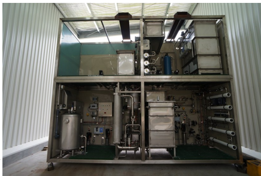
Advanced water treatment plant: bottom left – ozone and ceramic membranes; bottom right – BAC and RO; top right – UV, calcite contactor and chlorination; top left – laboratory and chemical storage.
